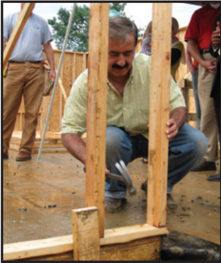
Homeowner Azad Saeed secures the first wall of his home on Manchester Road—the site of Joe Hodson's first Habitat volunteer experience.
